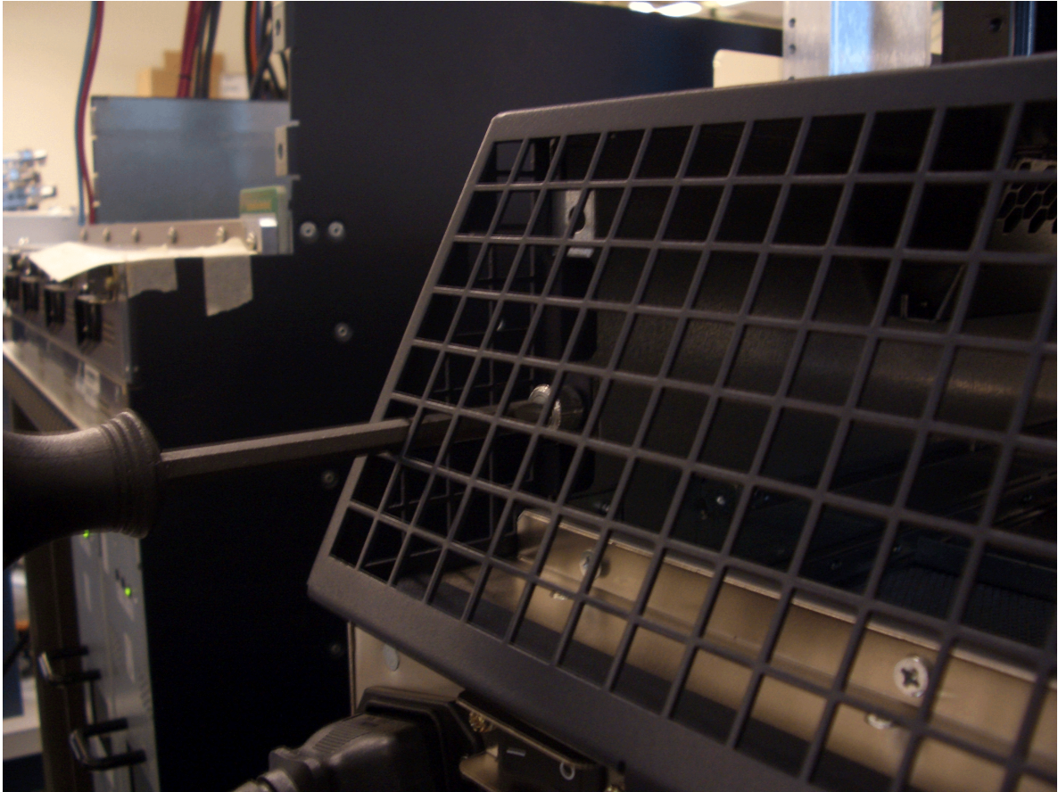
Figure 85: Removing the Left Captive Screw of the Rear Air Exhaust Grate
